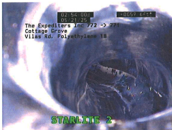
772-771_db0cff94-629b-4344-87d7-e5554e255330_20250521_152629_259.jpg, 00:03:02, 59.60ft Miscellaneous Survey Abandoned / Pipe Bends Down/Sag
