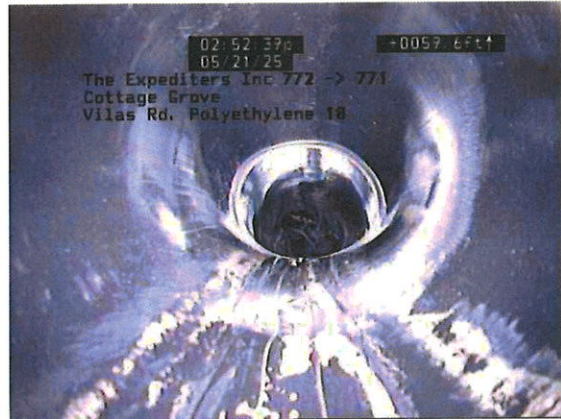
772-771_f7db0c77-7273-49a5-af2d-37f1addcbb67_20250521_152509_136.jpg, 00:02:37, 59.60ft Deformed Flexible Elliptical, 10%
