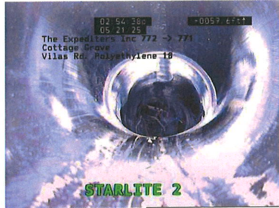
772-771_77cb5596-bd27-4455-8be5-f68d992f2f59_20250521_152707_760.jpg, 00:03:02, 59.60ft Miscellaneous Survey Abandoned / Pipe Bends Down/Sag
